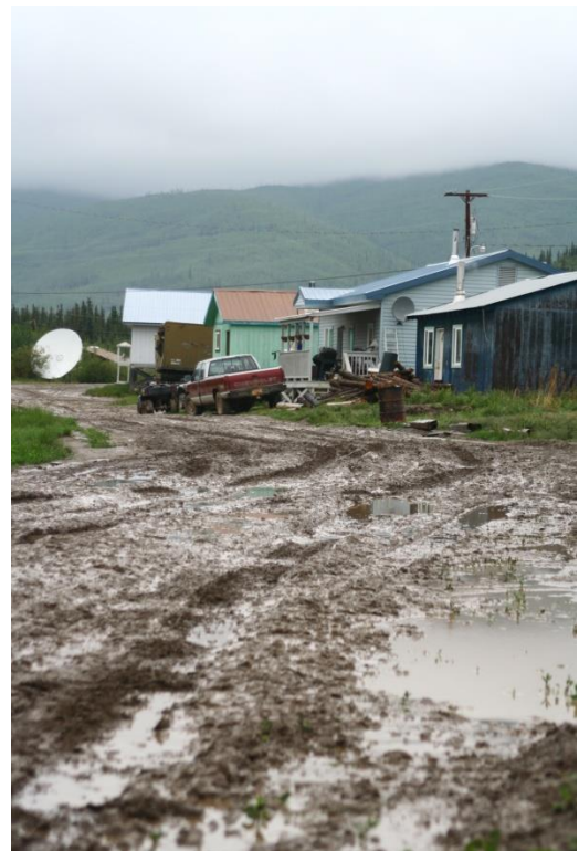
Figure 5: During heavy rains the road leading to Tetlin and roads within Tetlin become almost impassible with mud. Improving road conditions remains a high priority.
